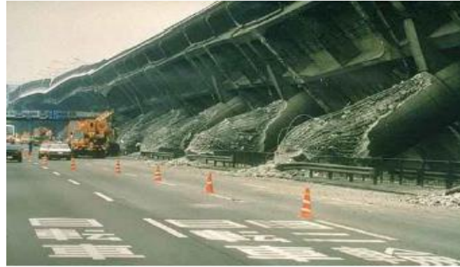
Figure 1.18 Collapse of the Hanshin Motorway, Kobe, Japan
